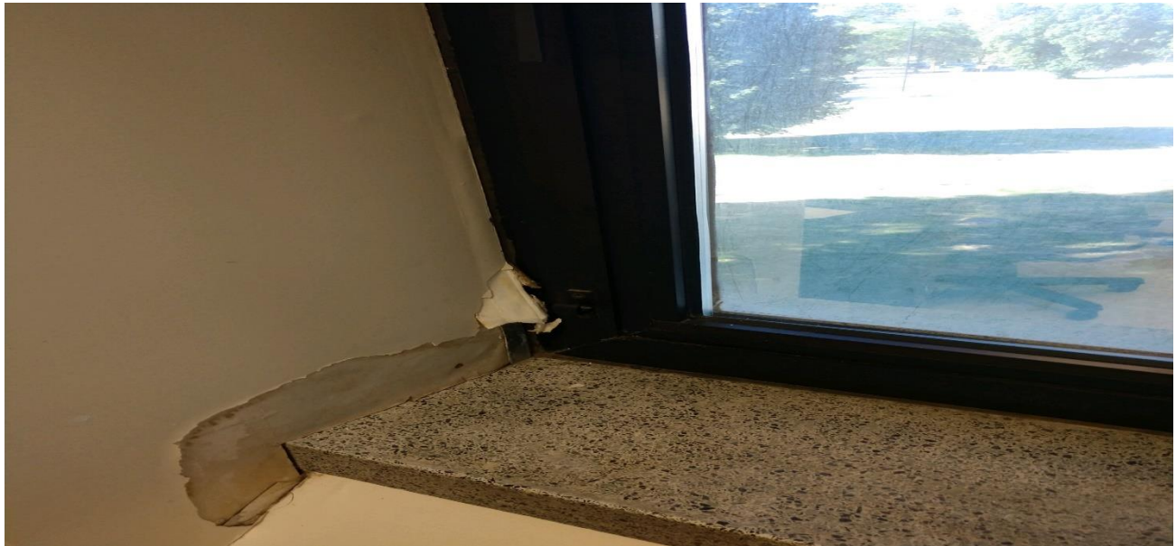
Martin Building Room 247, window damage
